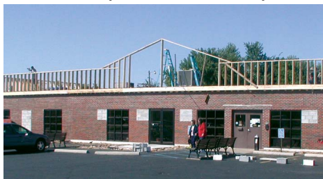
The brick front of the Loop was updated with a stucco facade and new roof line.
